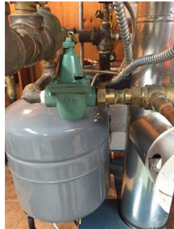
Isolated Fill Valve Component
