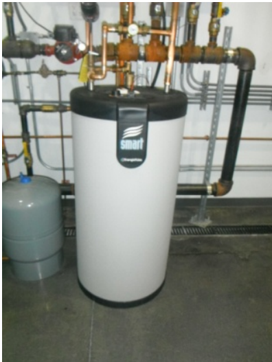
Overall photo of the SMART tank installation
