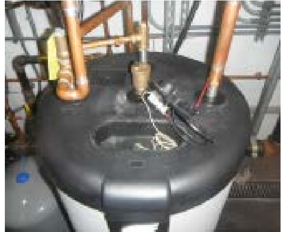
Top of the SMART tank showing connections and thermostat plate removed
